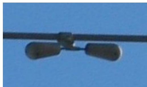
Figure 7: A Stockbridge damper, used to reduce vibration of overhead power lines
